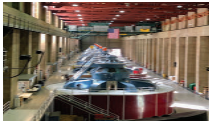
Generators inside Hoover Dam.
