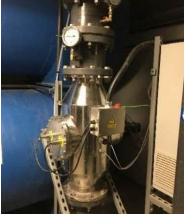
Figure 9: UV Water Treatment
